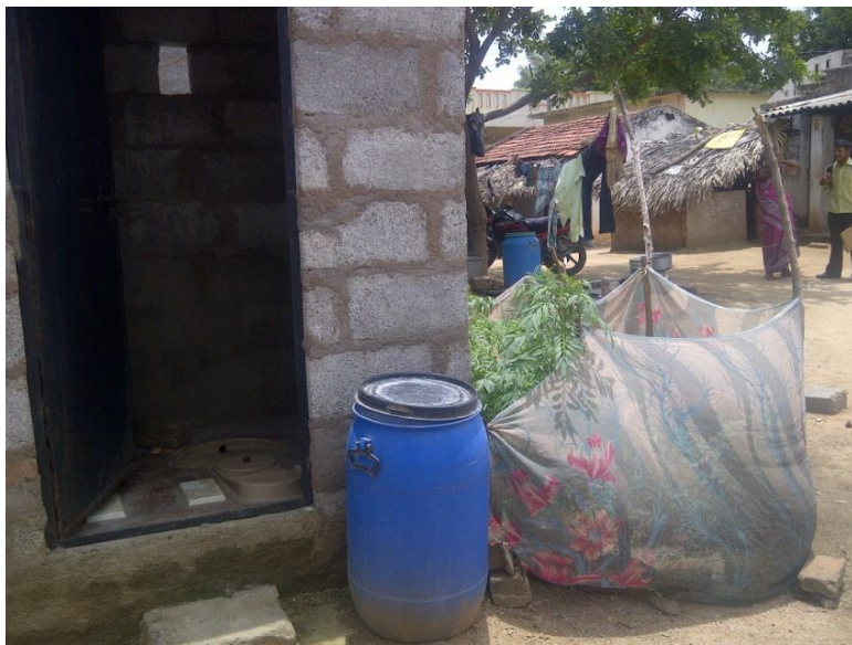
Eco sanitation toilet built by BDL
